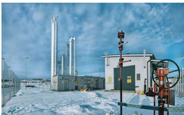
Figure 25: Biogas upgrading facility in Kujala, Lahti.
