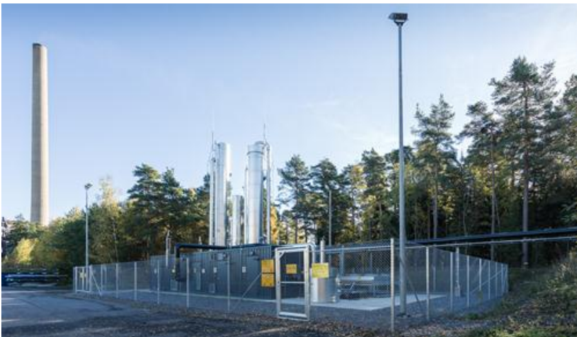
Figure 24: Biogas facility in Suomenoja, Espoo.
